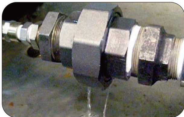
3000 lb MSS SP83 forged union with rusted sealing surfaces leaking with no pressure in the piping line. Once the sealing surfaces are rusted or compromised, they will always leak no matter how much torqued is applied
