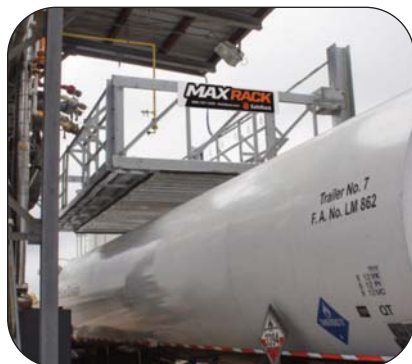
Chlorine gas unloading station
