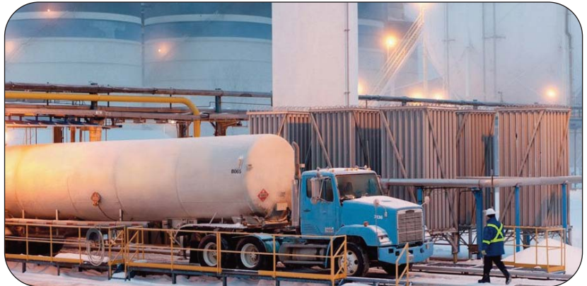
Tanker truck cryogenic bottom loading station
