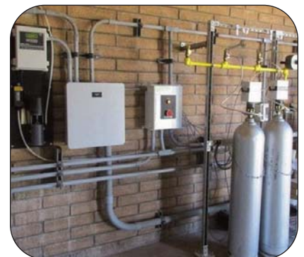
Chlorine gas feed system
